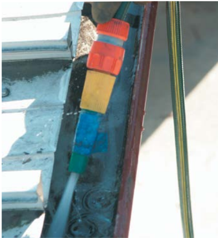
4) Rinse the gutter with water to soften and break up the dirt.
