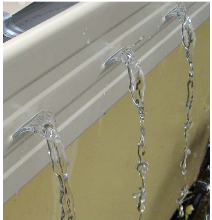
Typical overflow from slotted gutter.
